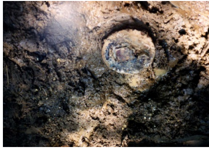
Figure 22. Borehole with contaminated water seepages
