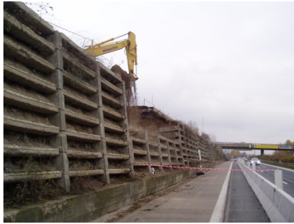
Figure 16. Original state of the retaining wall
