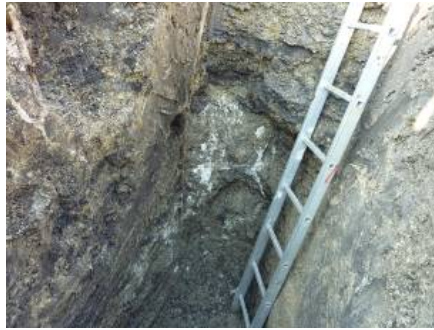
Figure 21. Grouting material in the surrounding of the water-gate (photo from the control excavation after 10 years)
